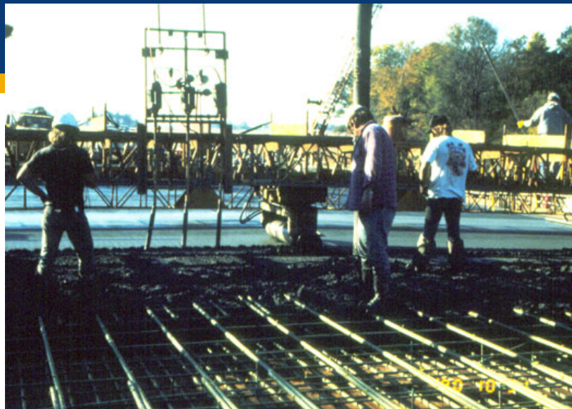
(Mud placement, Single Drum Screed, Gang Vibrators) (CHECK/RECORD Cover & Fillet Depths at 10 th
